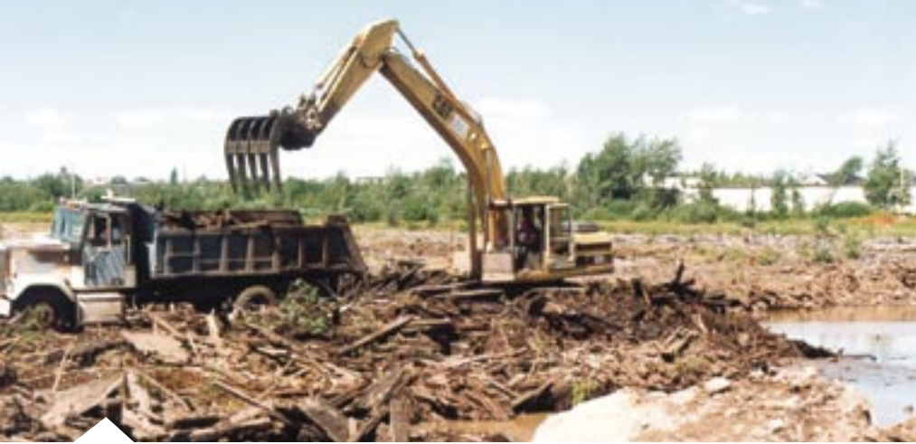
EXCAVATION OF LUMBER AND WOOD WASTE DISPOSAL AREA IN WESTERN SECTOR (RECLAIM YARD) OF FORMER CN RAIL CAR SHOPS PROPERTY (JULY 1997).
