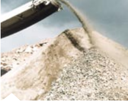
STOCKPILING OF CRUSHED CONCRETE TO BE RECYCLED AS ROADWAY BASE IN NEW DEVELOPMENT (JUNE 1998).
